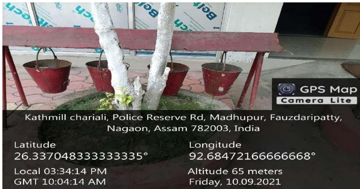
Figure 49: Fire Extinguisher Bucket
