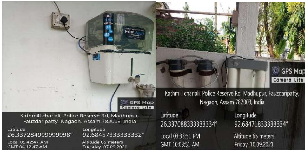
Figure 44: Drinking Water Facility
